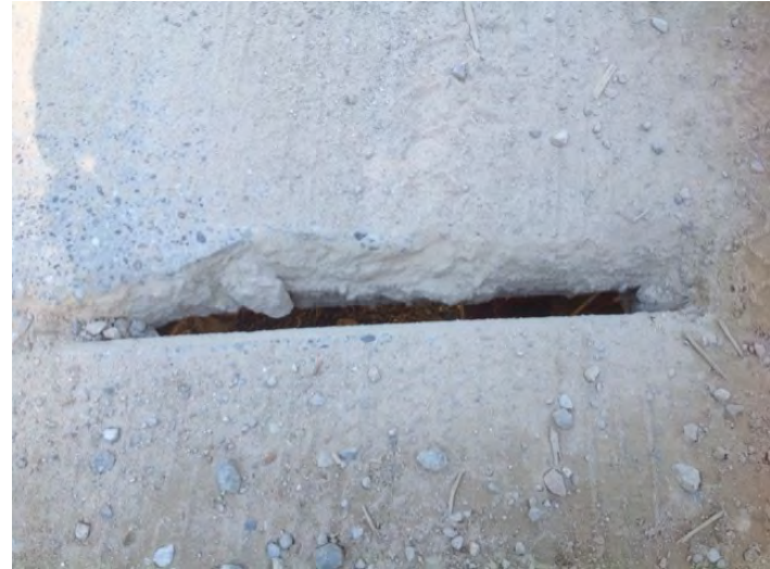
panel damage on left approach
