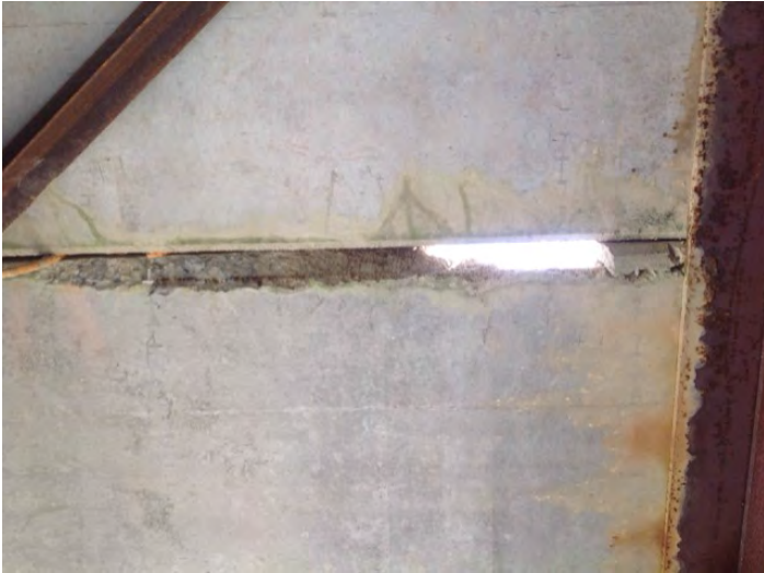
deck panel damage from underneath
