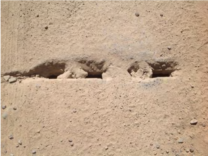
panel damage right approach
