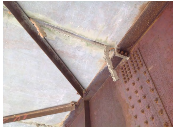
deck seals all falling out
