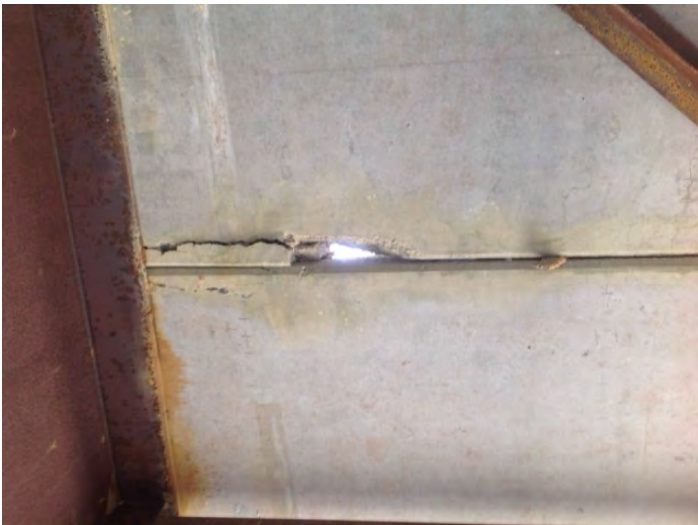
deck panel damage from underneath
