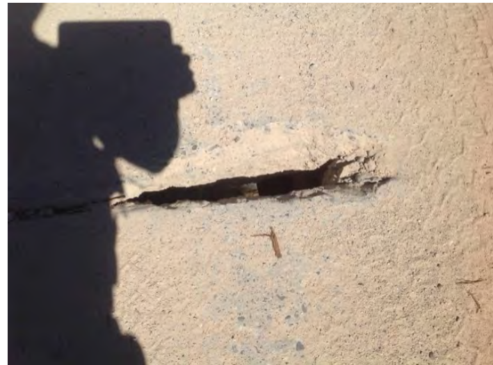
panel damage mid span
